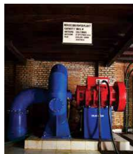
Mini-hydro power plant - Battalgalla
